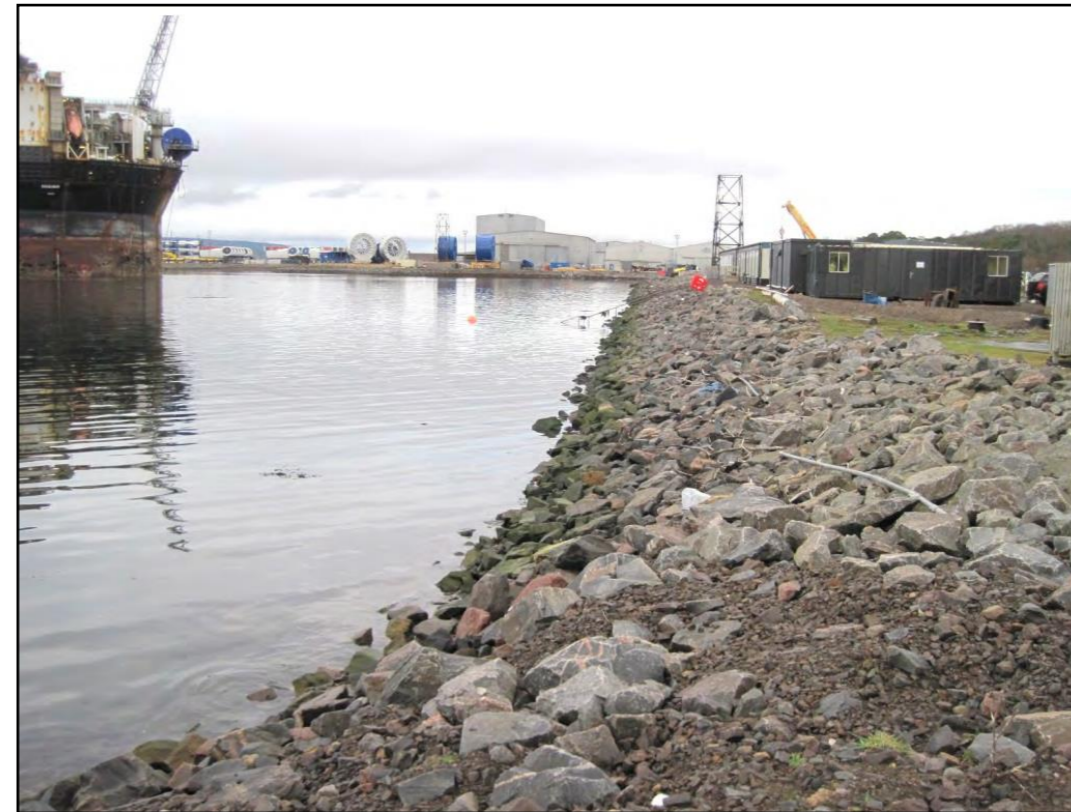
Plate 2-1: View of the existing revetment on east side of the Inner Dock looking north
